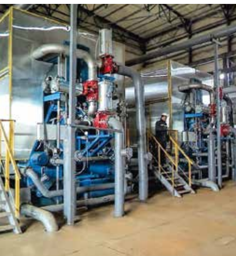
Membrane filter presses
